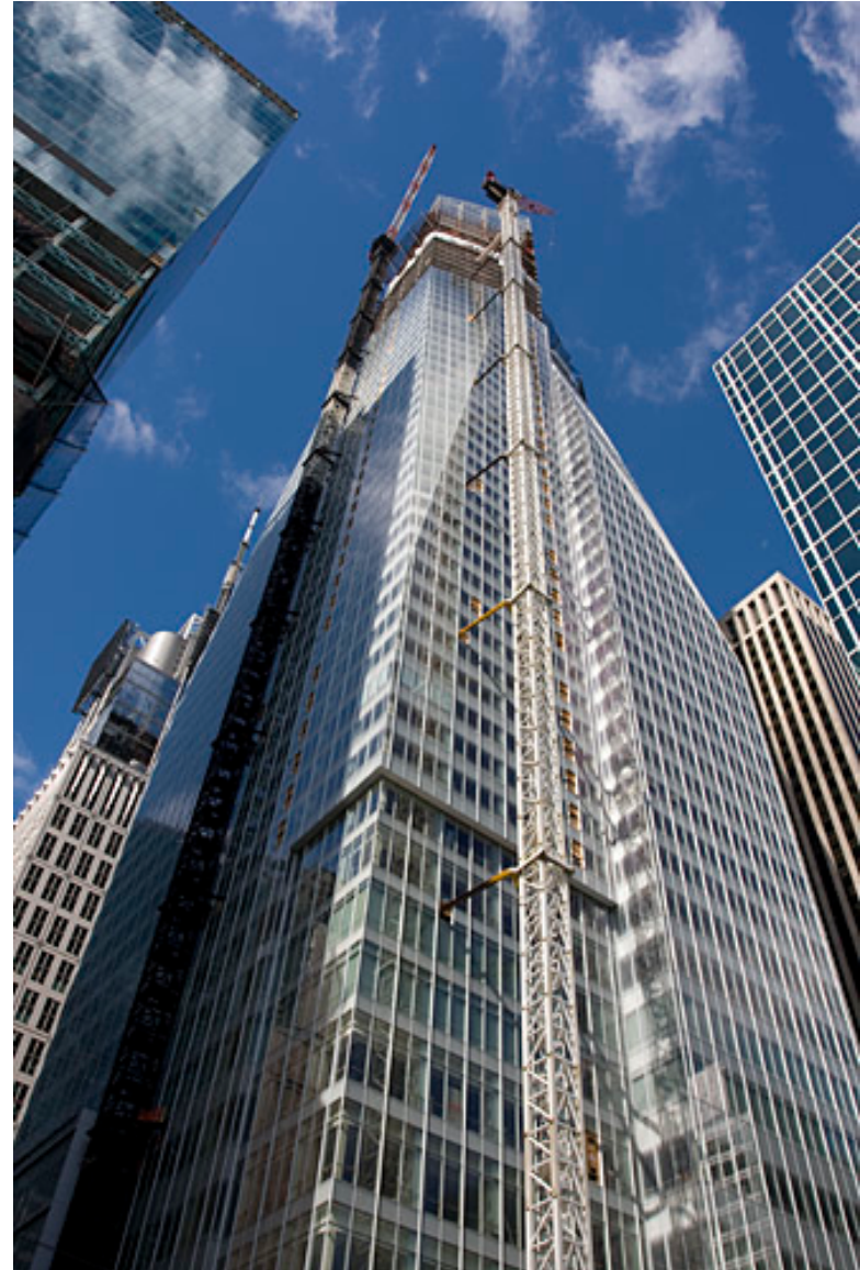
BANK OF AMERICA TOWER, NYC, LEED PLATINUM
